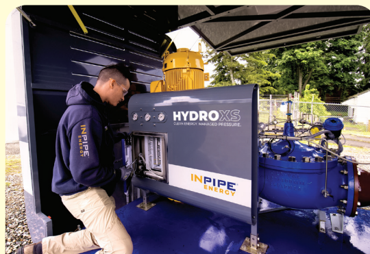
An InPipe Energy technician works on the HydroXS energy recovery system at Skagit PUD's 9th and Highland reservoir site.
