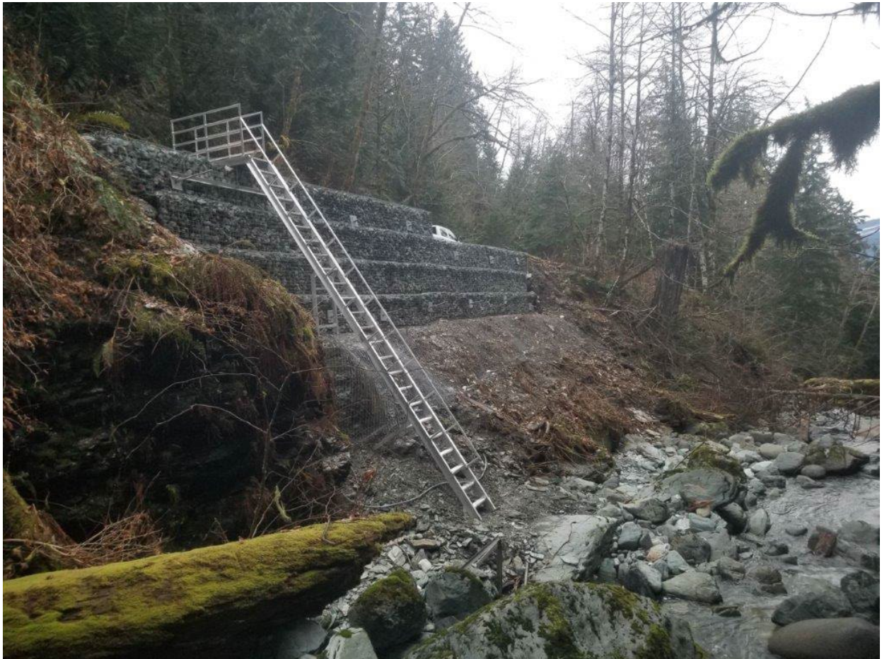
Figure 2-10b. Gilligan Creek Roadslide Repair at Intake
